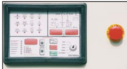
Example of DST4600 AMF Panel
